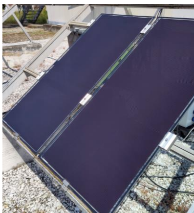
Figure 14. The two-perovskite mono-junction solar modules in the ESTI outdoor monitoring site.
