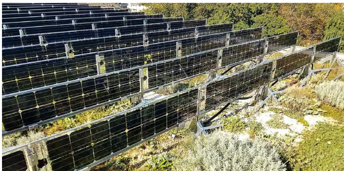
Figure 16. Vertical bifacial PV system on green roof.
