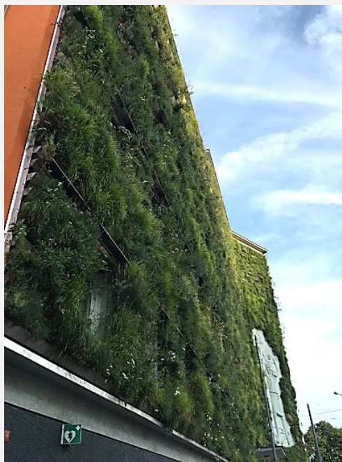
Pilot Green wall on MA48 (© Vera Enzi)
