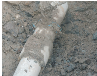
Image: Contaminated soil around deteriorated asbestos-cement pipe.
